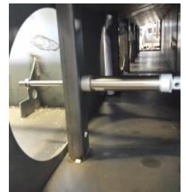
Fume extraction valves
